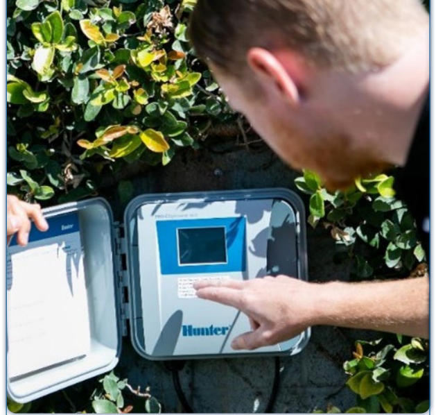
Customer’s value smart controllers with remote access.
