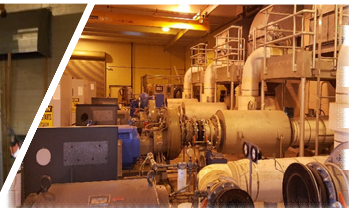
CCWRP Existing Blowers
