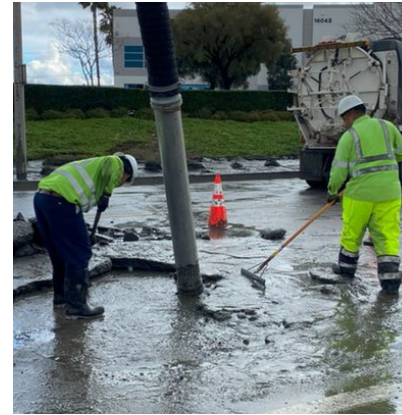
Broken asphalt caused by rupture
