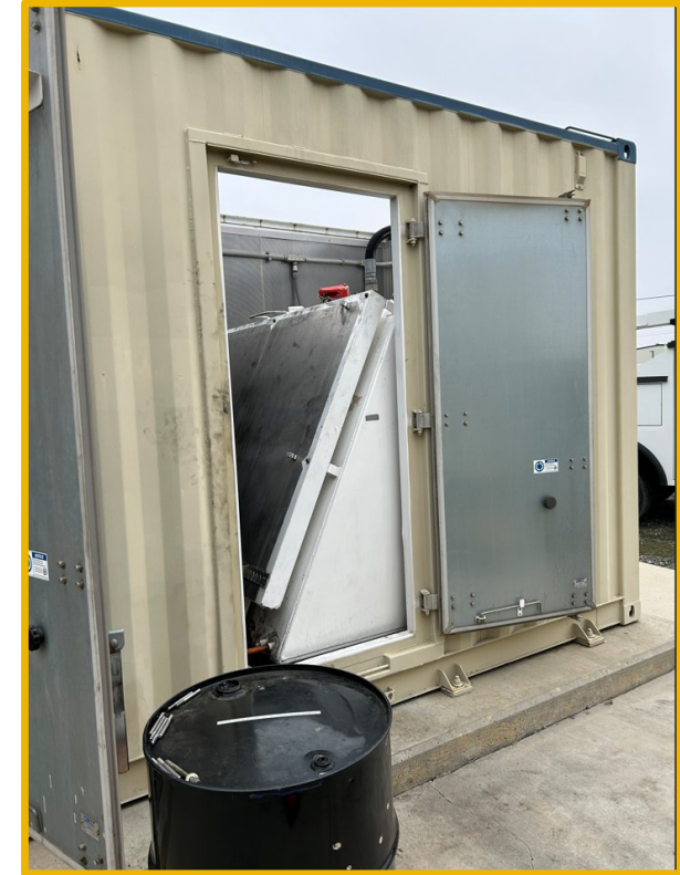
New Unit Installed
