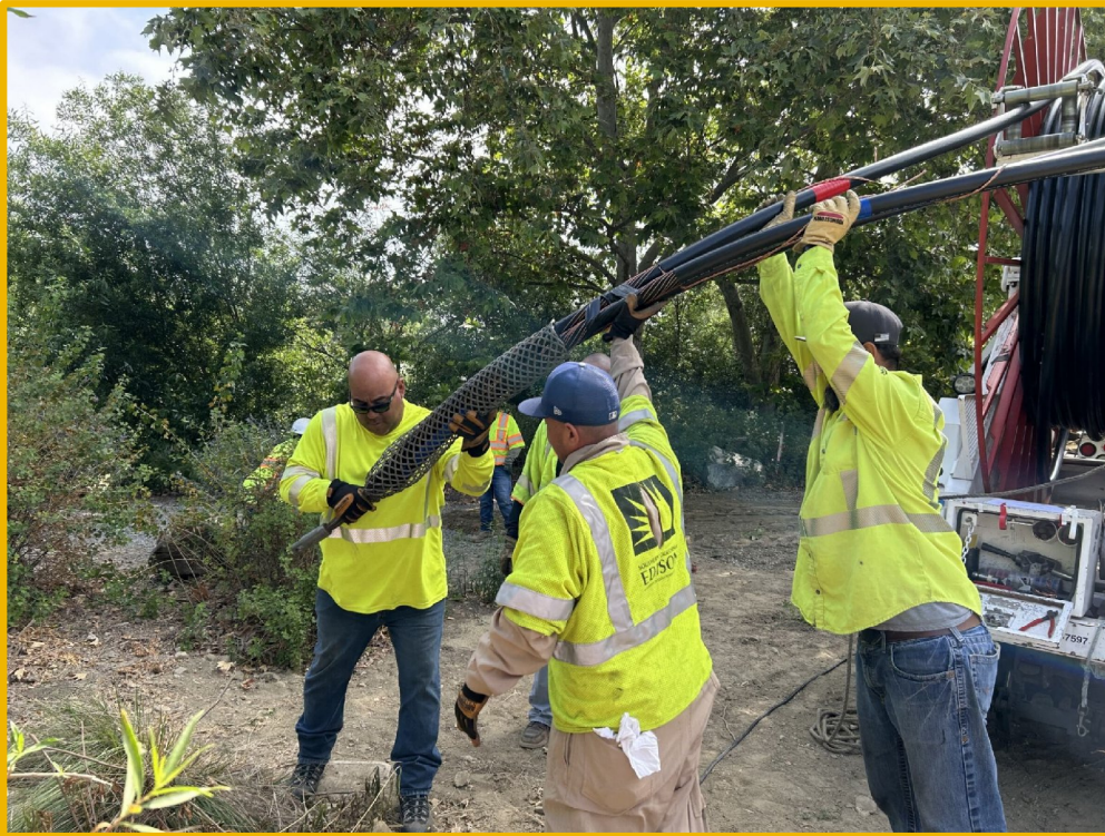
Park Vault in Park to Pole: 180'
