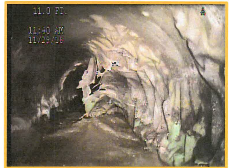
Cucamonga Trunk Sewer Coating Failure
