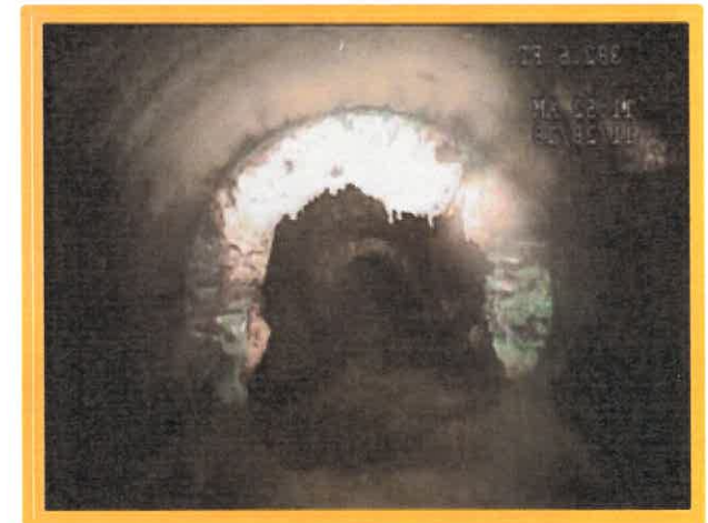
Cucamonga Trunk Sewer Coating Failure
