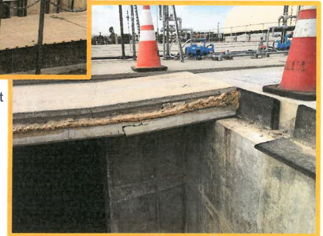
Concrete Cover Failure
