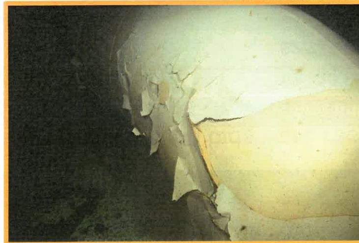
Coating Delamination on Piping
