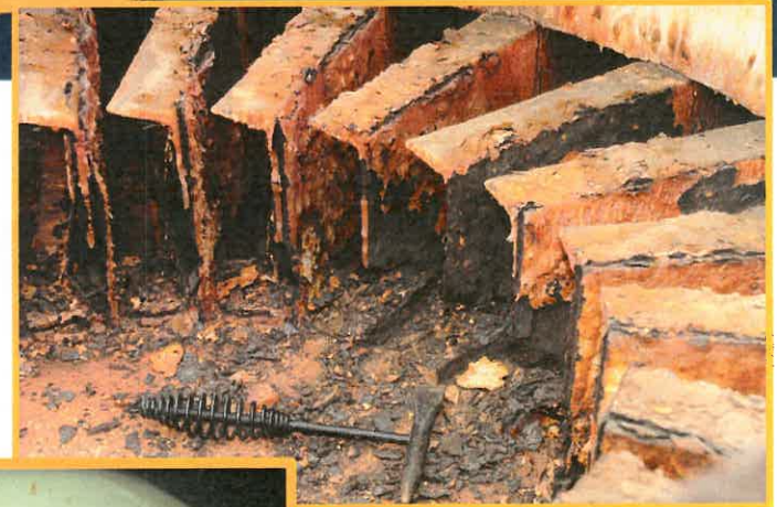
Corrosion Damage on Rafters
