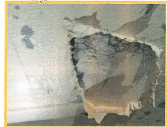
Failed Internal Roof Coating
