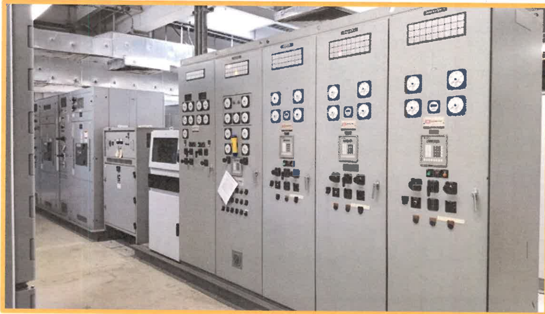
RP-1 Emergency Generators
