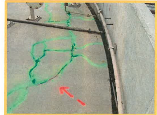
Digester No. 6 Partial Roof Cracks
