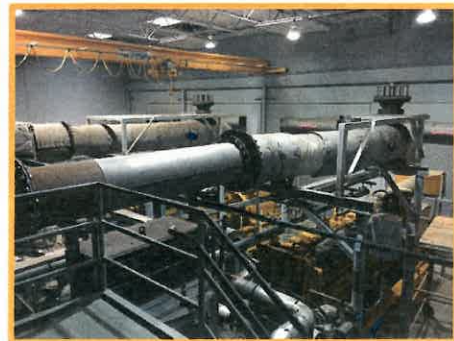
REEP Exhaust Piping
