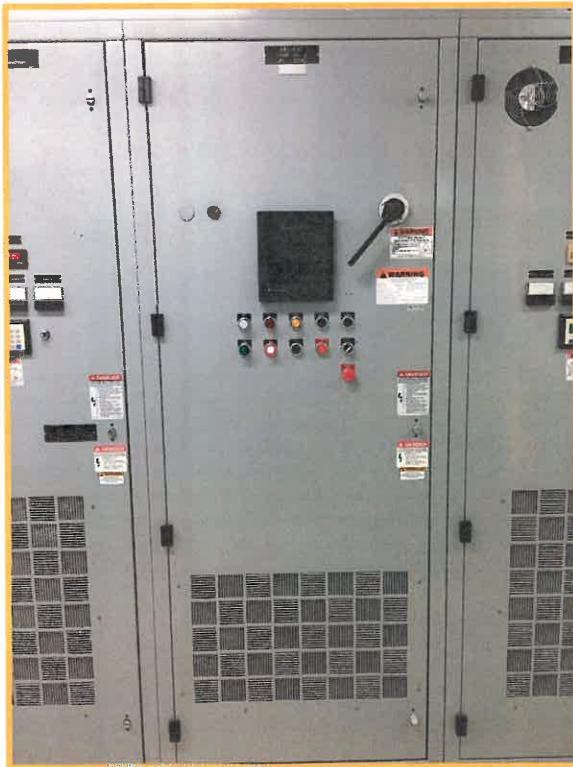
Influent Pump Control Center
