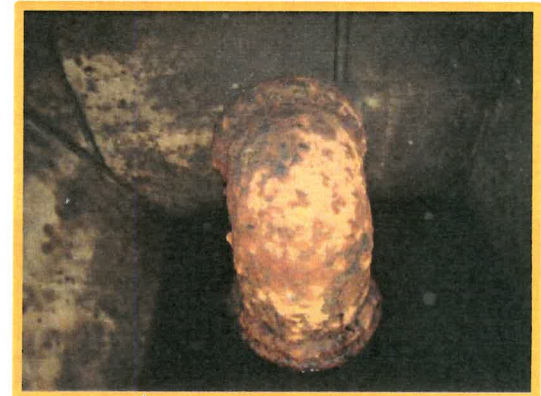
Corroded pipe in pump station wet well
