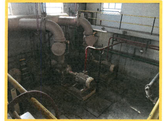
Obsolete pumps, equipment, and piping
