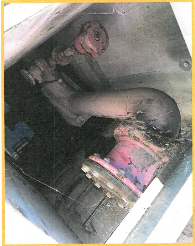
Existing Air Vac in Vault
