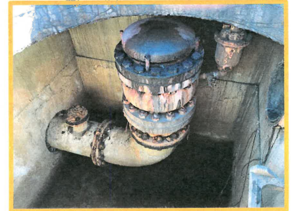
Existing Air Vac in Vault
