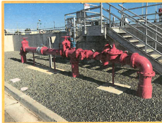
RP-5 Recycled Water Piping
