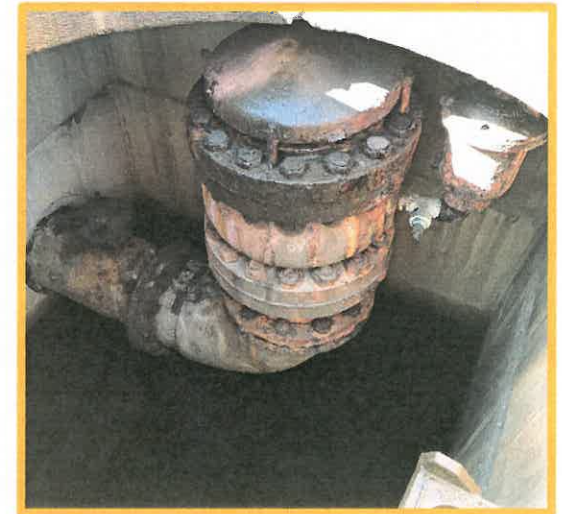
Existing Combination Air Relief Valve
