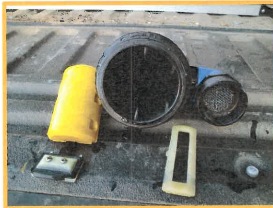
Inside existing A.R.I. Valve
