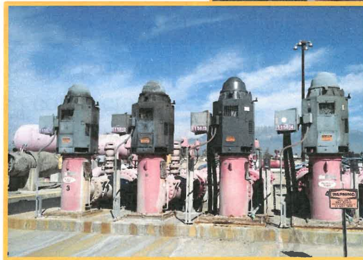
RP-1 Recycled Water Pump Station
