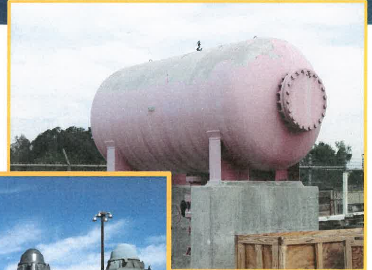
Existing 2,500 Gallon Surge Tank
