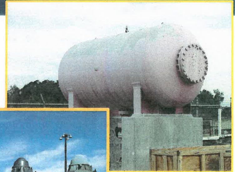
Existing 2,500 Gallon Surge Tank
