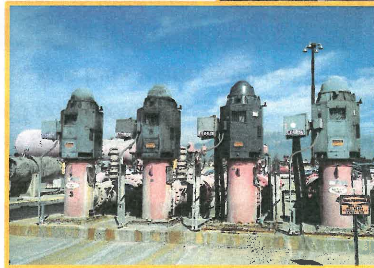
RP-1 Recycled Water Pump Station
