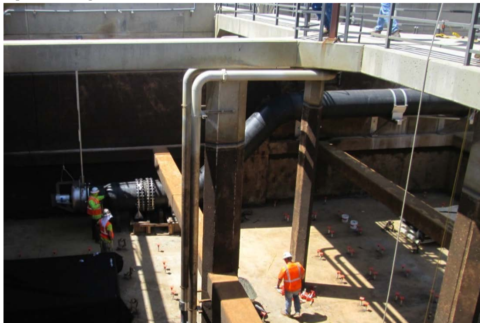
The performance of the RP-1 mixed liquor return pumps were adjusted to run at optimal rates.
