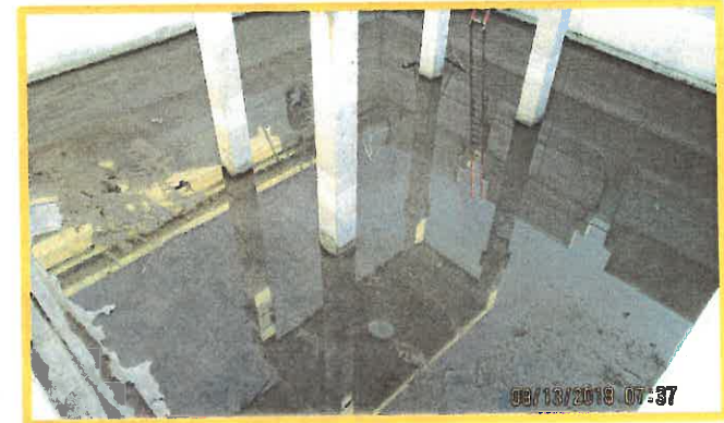
Ground Water Infiltration 09/13/18 7:37 AM
