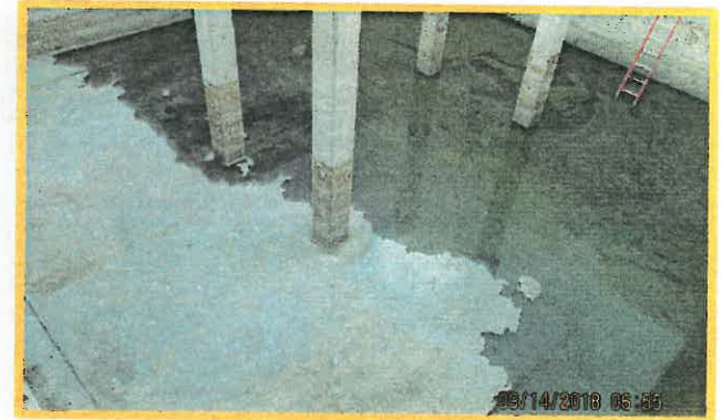
Ground Water Infiltration 09/14/18 6:55 AM
