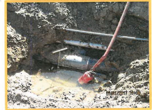
RW Pipe Rupture Repair Due to Surge
