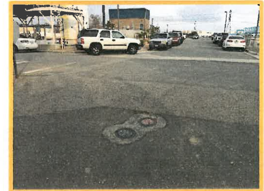
Sample Location - Non-Functional Buried Isolation Valves
