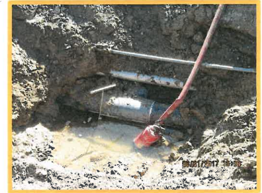
RW Pipe Rupture Repair Due to Surge
