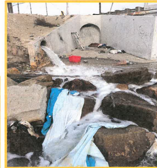
Existing Recycled Water Discharge
