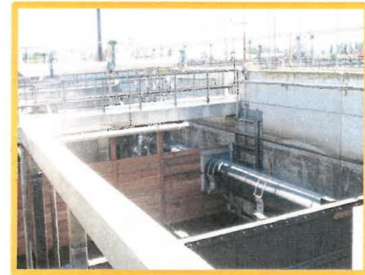
Baffle Walls and Mixed Liquor Return Pumps
