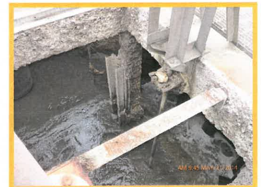
Distressed Diversion Structure
