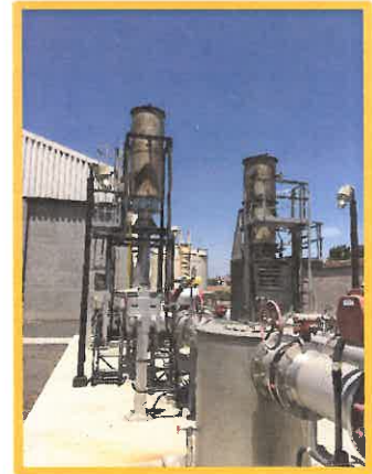
Aereon Flares – City of Riverside
