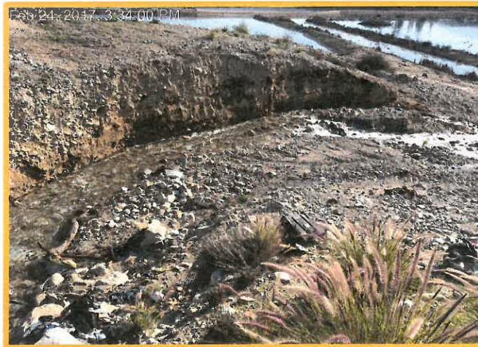
Existing Erosion in Unlined Channel
