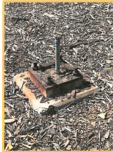
Existing Damaged Base
