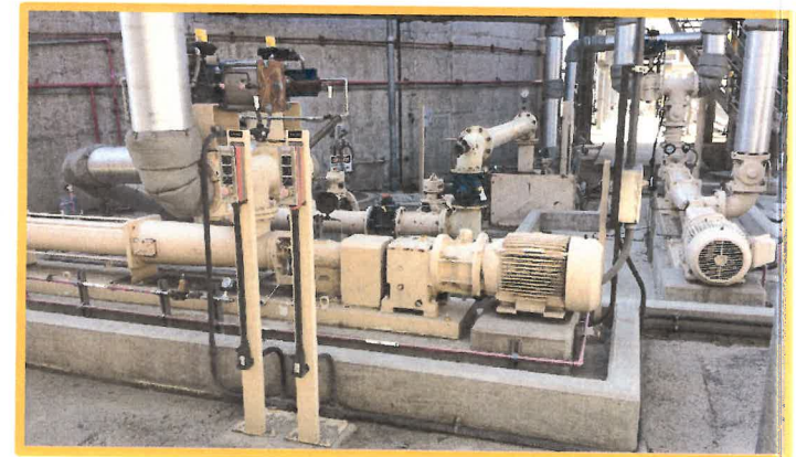
Sludge Transfer Pump at Digester Area
