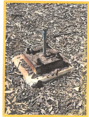
Corroded Light Pole at RP-1
