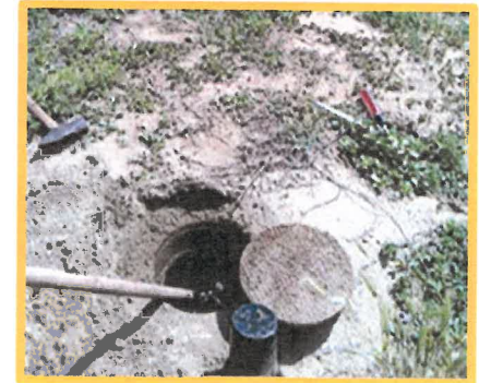
Cathodic Protection Test Stations
