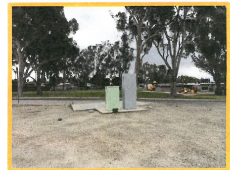
Vault with Valve
