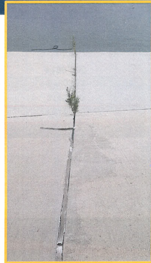
Failed Expansion Joint Sealant
