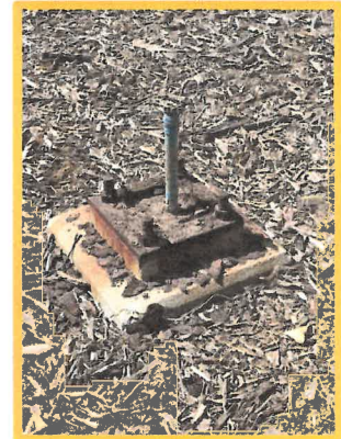
Corroded Light Pole at RP-1
