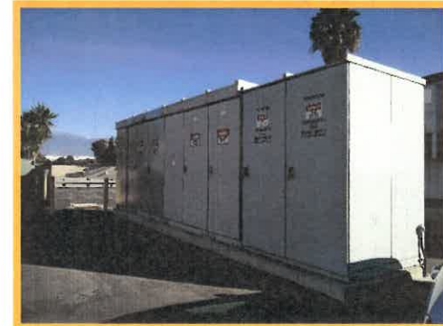
Two 12kV Switchboard Sections Will Be Added
