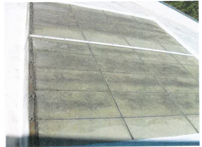
Discolored and Deteriorated Skylight
