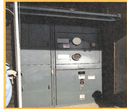
480V Switchgear To be Replaced
