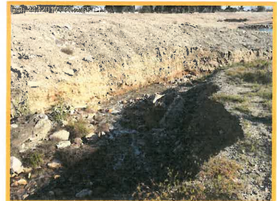
Eroded Slopes at Unlined Channel
