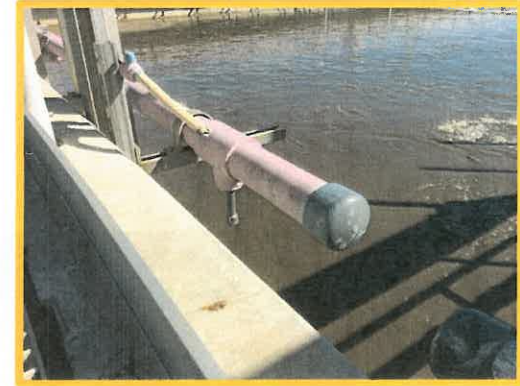
Out of Service Surface Sprayer Pipeline
