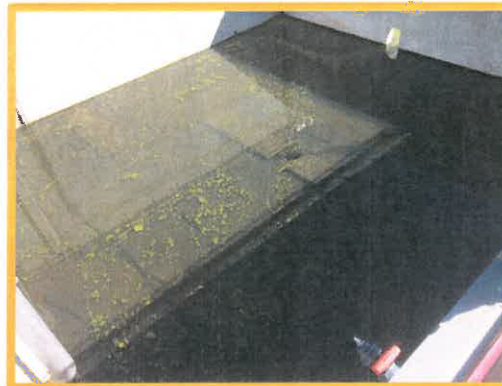
RP-5 Aeration Basin with Failed Diffusers
