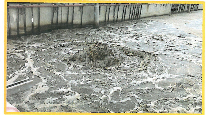
Aeration Basin Surface Boil
