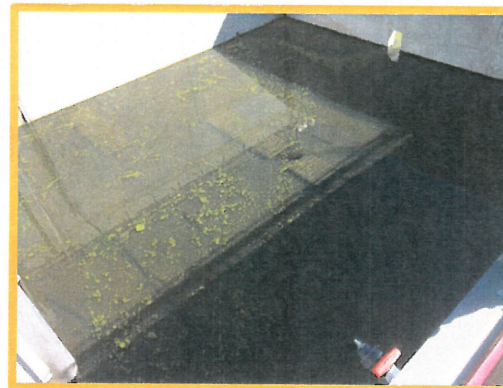
RP-5 Aeration Basin with Failed Diffusers
