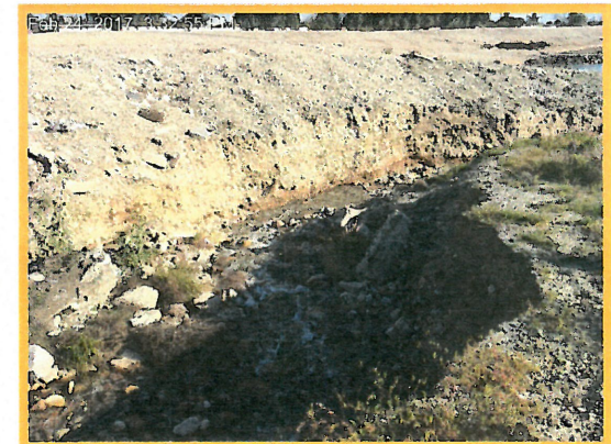
Eroded Slopes at Unlined Channel
