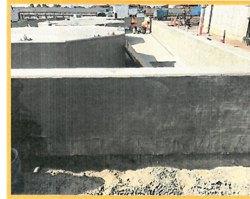
New Chemical Area with Tank Pad
