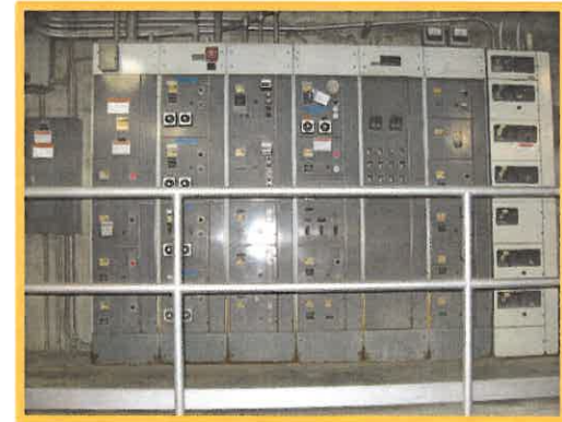
Obsolete Electrical Components
