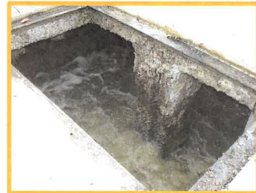
Corroded Concrete Deck
