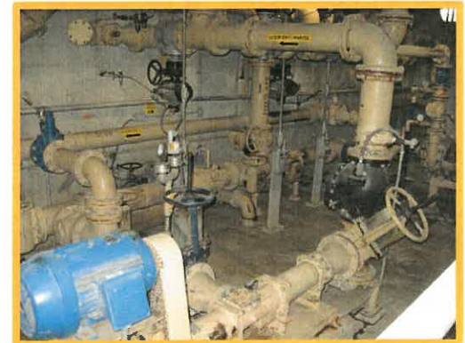
Existing Scum System
