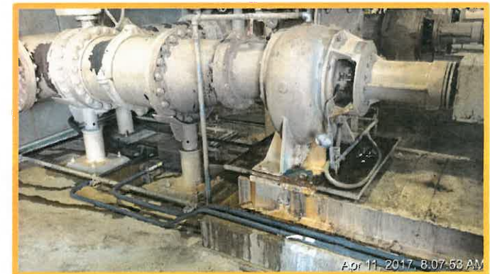
RAS Pump at End of Useful Life
