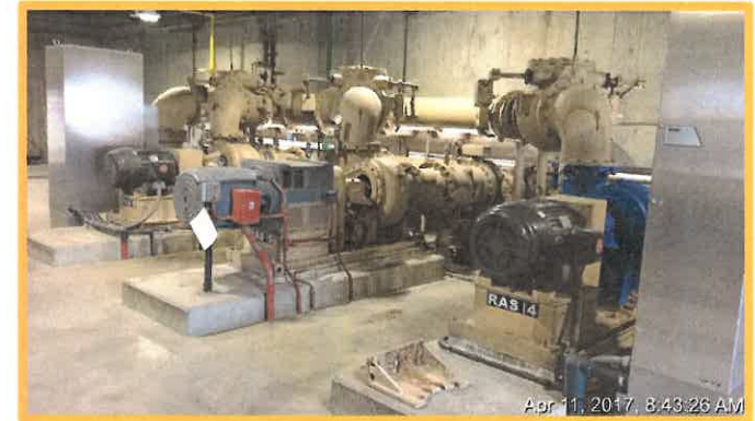
RAS Pump Equipment and Appurtenances
