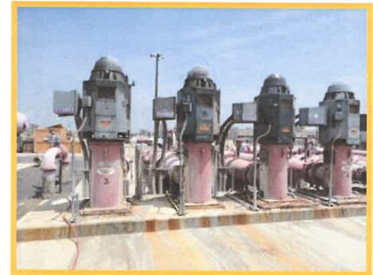
Recycled Water Pump Station Motors
