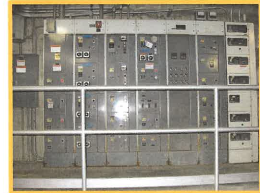
Obsolete Electrical Components
