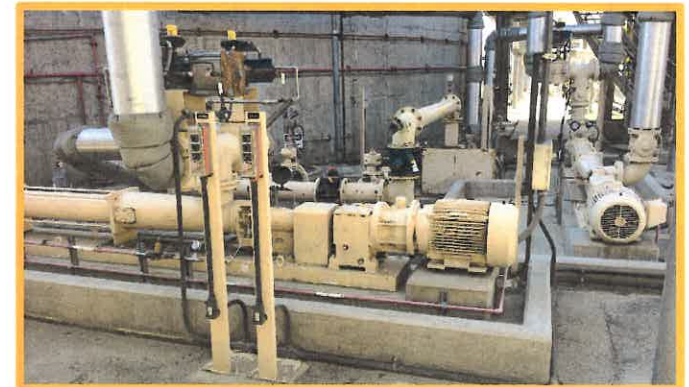
Digester Transfer Sludge Pump Clogging
