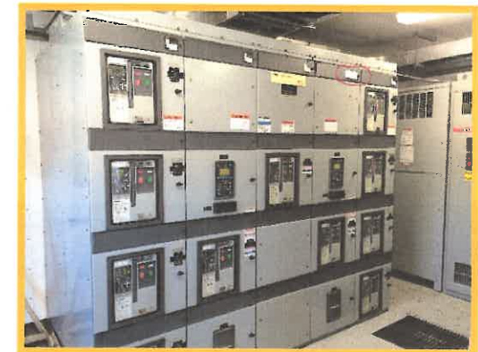
Front of Switchgear
