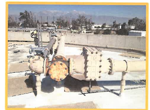
Digester No. 6 Flame Arrestor
