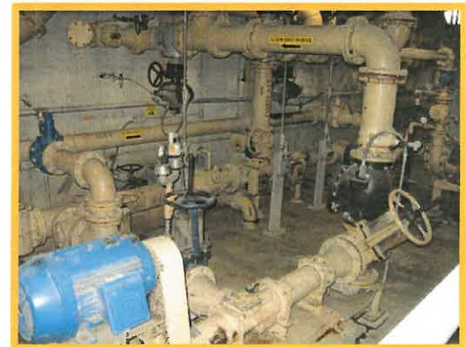
Existing Scum System
