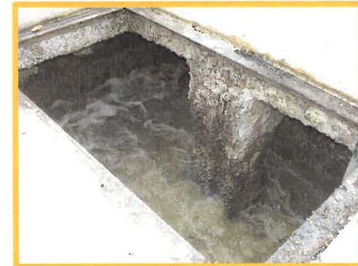
Corroded Concrete Deck
