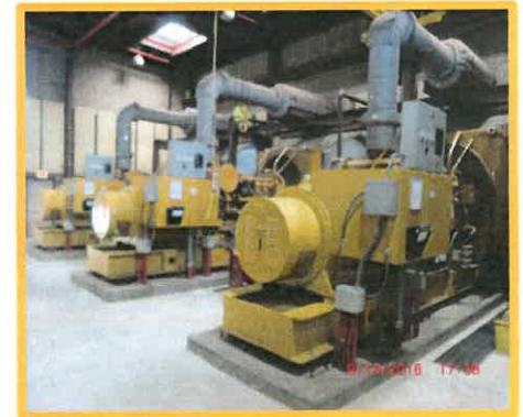
Back up Generators at RP-1
