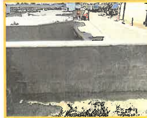
New Chemical Area with Tank Pad
