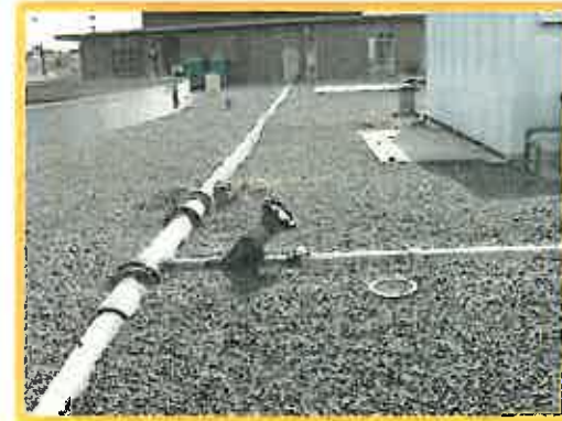
Existing Line at RP-1
