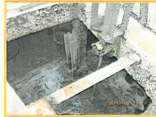
Exposed Rebar In Grating at Support Beam
