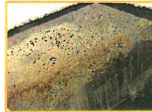
IPS Wet Well Concrete Corrosion
