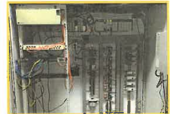
Typical Control Panel Interior
