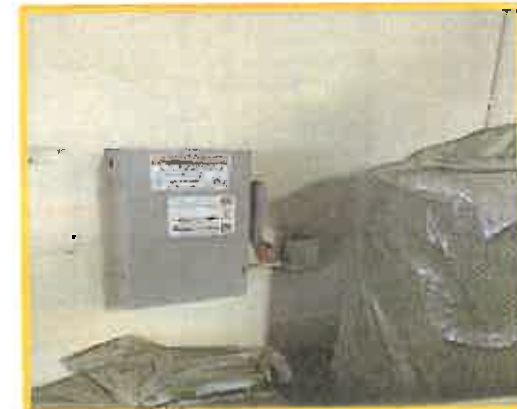
Disconnect to be Removed
