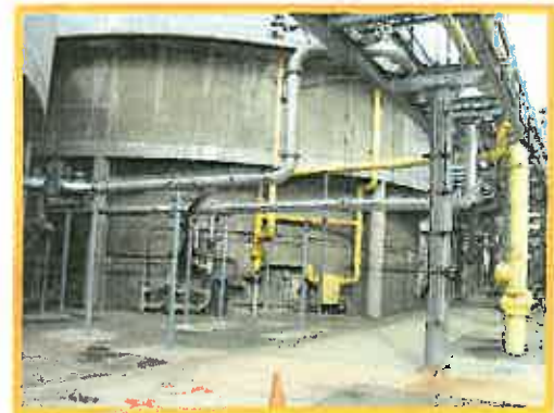
Above-Ground Connection at Digester 1
