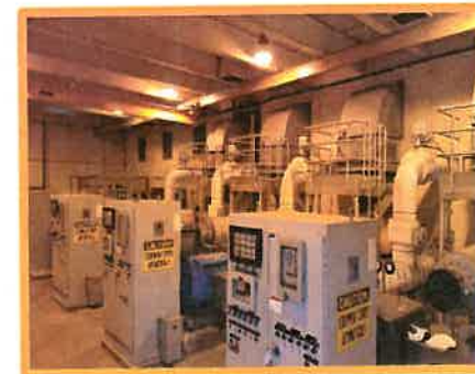
Aeration Blowers and Controls
