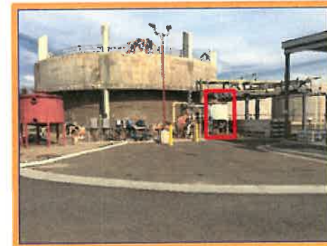
Acid Phase Digester Iron Sponge
