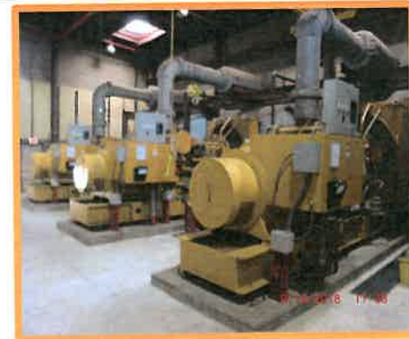
Back up Generators at RP-1
