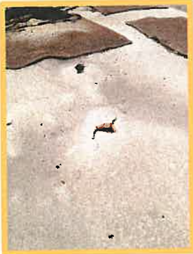
Cracking of Foam Roofing Insulation
