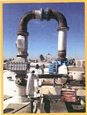
Gas Mixing System on Digester Roof
