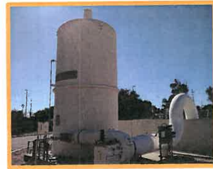
Existing Odor Control Vessel
