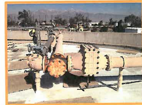
Digester No. 6 Flame Arrester
