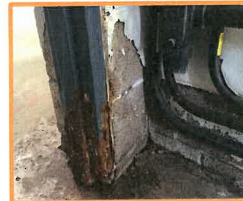
Corrosion from Bleach Leakage at Existing Tanks
