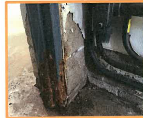
Corrosion from Bleach Leakage at Existing Tanks
