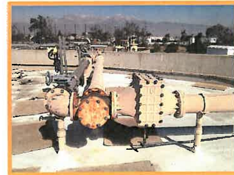
Digester No. 6 Flame Arrester
