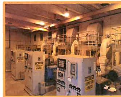
Aeration Blowers and Controls
