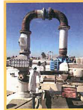
Gas Mixing System on Digester Roof
