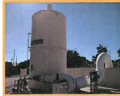
Existing Odor Control Vessel
