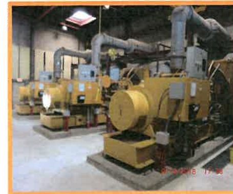
Back up Generators at RP-1
