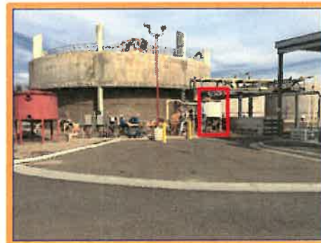
Acid Phase Digester Iron Sponge
