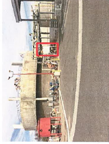
Acid Phase Digester Iron Sponge
