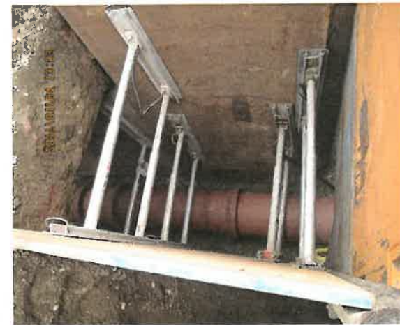
18-in Pipeline Between Manholes
