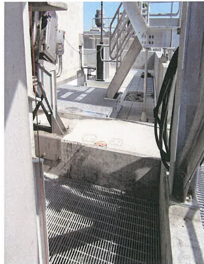
Potential Tripping Hazard
