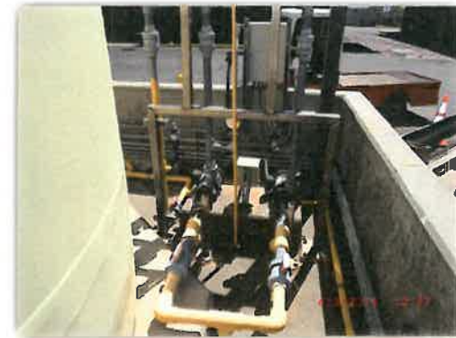
Bleach Loop Pumps
