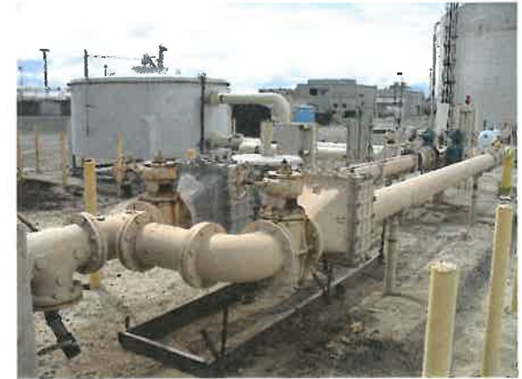
Digester Gas Piping to the Flare
