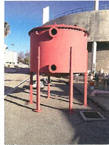
Acid Phase Digester Iron Sponge
