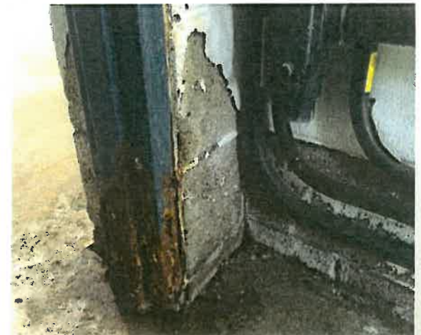
Corrosion from Bleach Leakage
