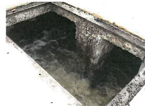
Corroded Concrete deck
