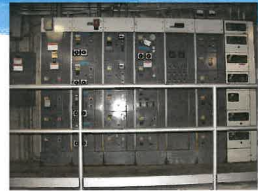
Obsolete Electrical Components in Primary Gallery
