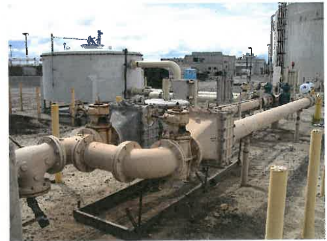
Digester Gas Piping To The Flare
