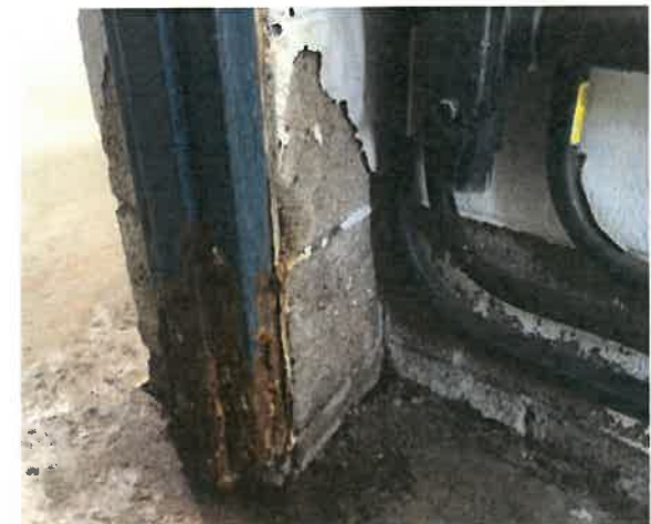
Corrosion from Bleach Leakage
