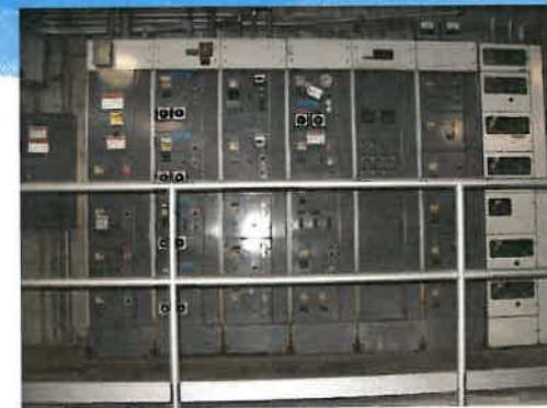
Obsolete Electrical Components in Primary Gallery
