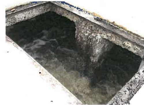
Corroded Concrete deck
