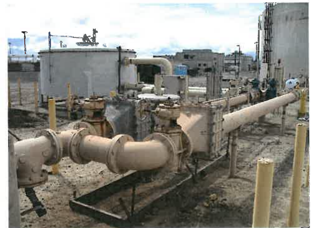
Digester Gas Piping To The Flare
