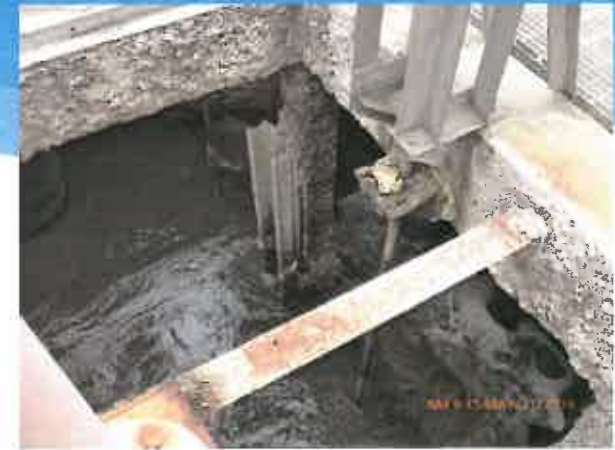
Exposed rebar in grating in support beam
