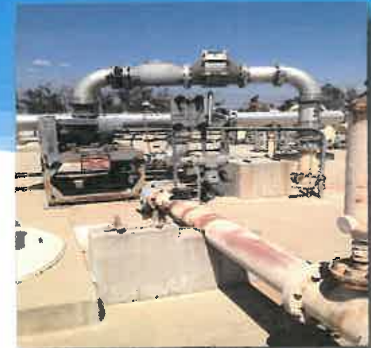
Gas Mixing System on Roof
