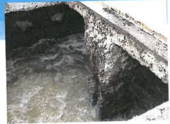
Concrete Degradation at RP-1 Headworks
