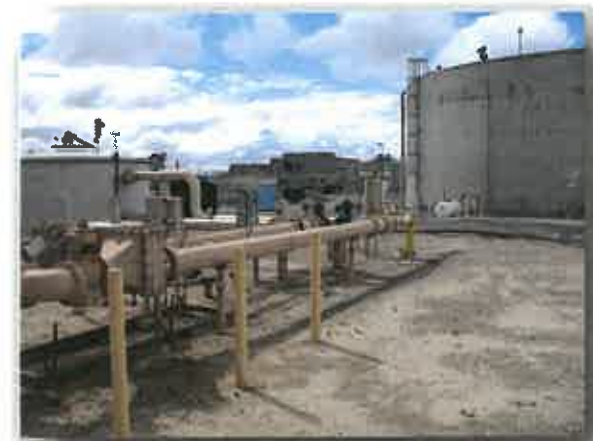
RP-1 Flare Gas Piping
