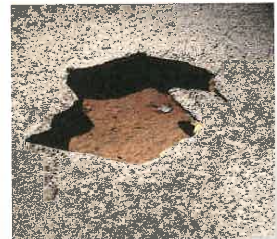
Digester Roof Foam Spray Damage
