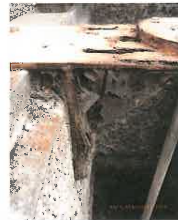
Valve Stem Support Bracket Corrosion
