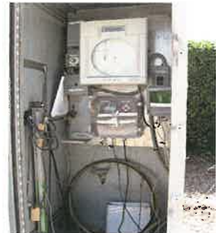
Existing Electrical Panel
