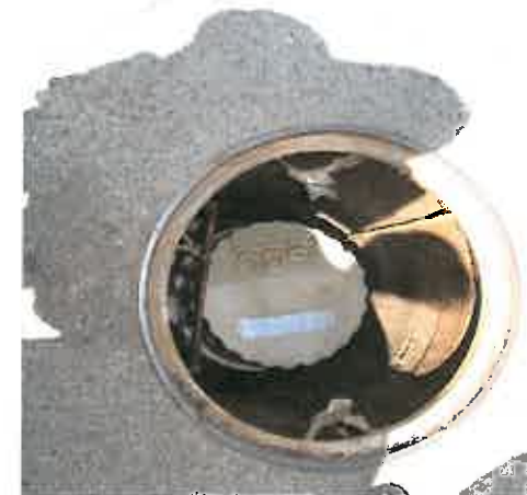
Existing Sampling System
