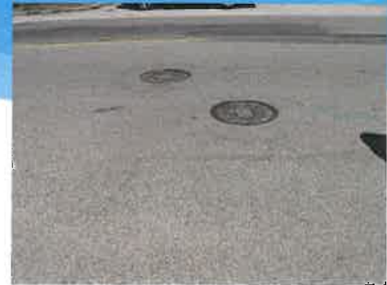
Flow meter and sampling manholes
