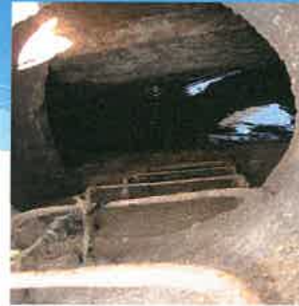
42 inch NRW line with flume flowmeter
