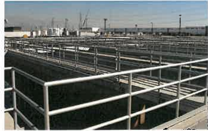
Chlorine Contact Basin (CCB)
