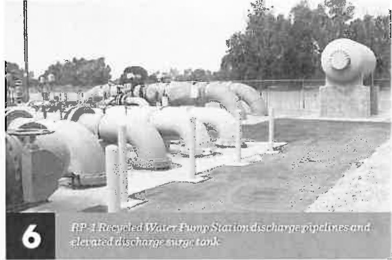
RP-1 Recycled Water Pump Station elevated discharge surge tank
