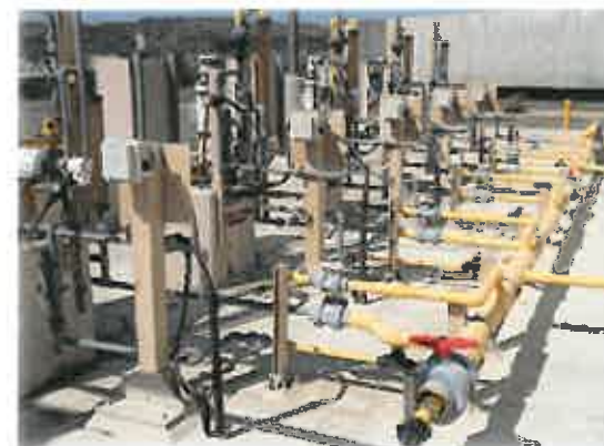
Sodium Hypochlorite Chemical Pumps
