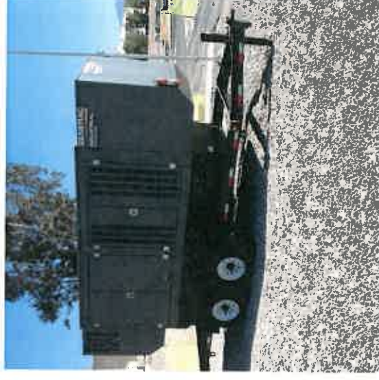
Existing Portable Generator
