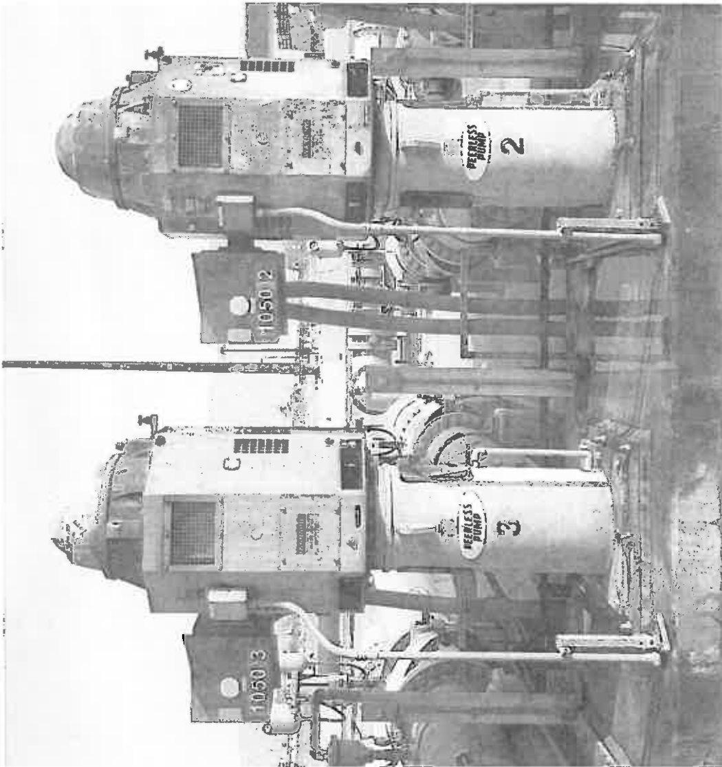
RP-1 1050 Pressure Zone Pumps No. 2 & 3
