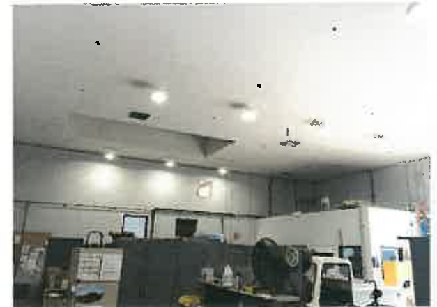
Interior Lighting at RP-4 Warehouse
