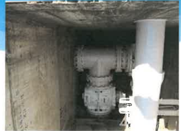
One of two 18" valves in DAFT Valve Vault No. 1
