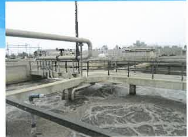
RP-1 Aeration Basins
