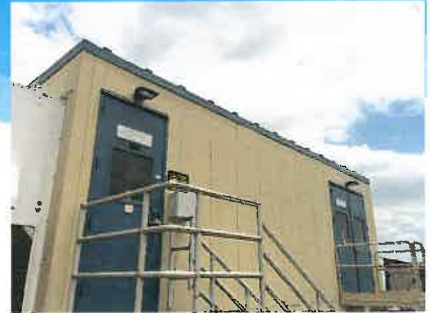
Exterior Lighting at MCC Building
