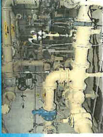
Scum Pump Location
