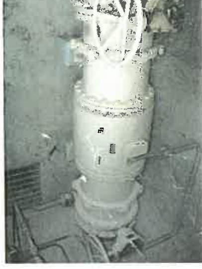
System C Flow Meter
