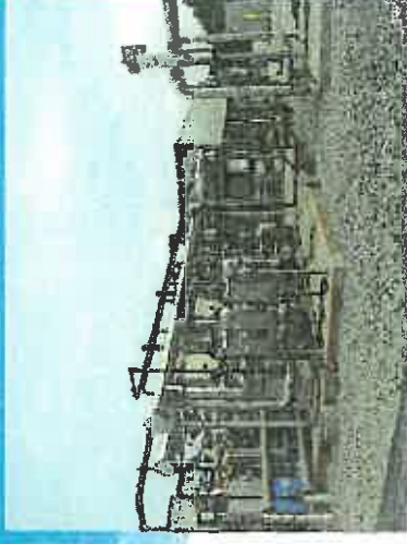
Central Chiller Plant
