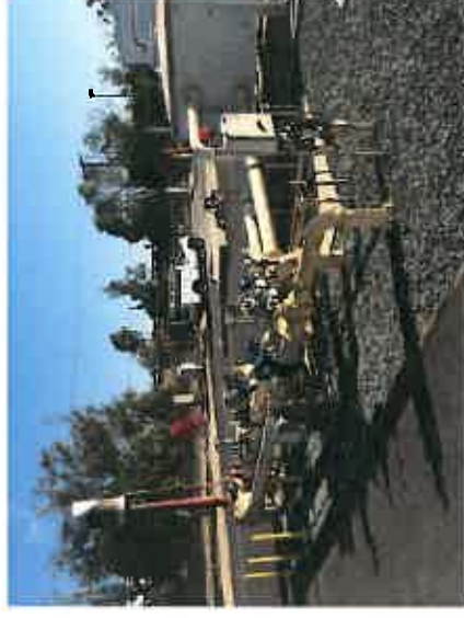
New PRV and Bypass Piping
