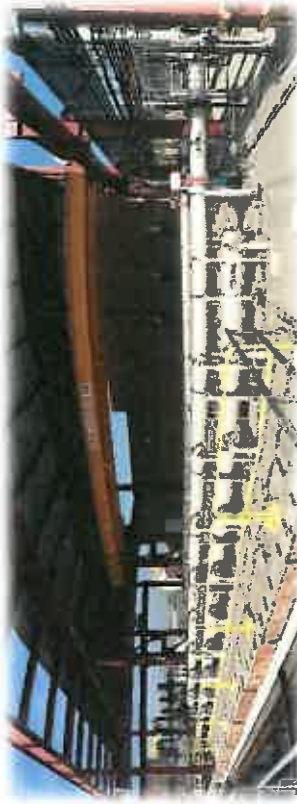
Riverside Water Quality Control Plant MBR System – Online March 2016
