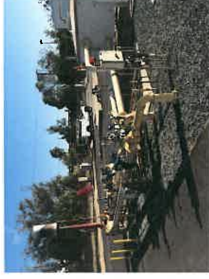
New PRV and Bypass Piping
