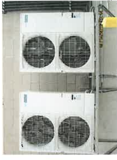
RP-2 Dewatering Building Control Room Condenser Units
