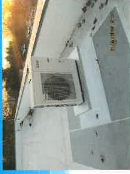
Condenser Unit at RP-5 Control Room
