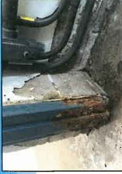
Corroded Existing at Chemical Building
