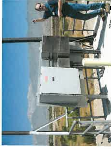
Radio Cut-Over from Old to New System
