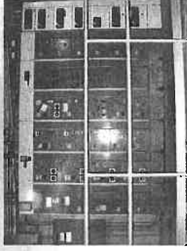
Obsolete Electrical Components in Primary Gallery
