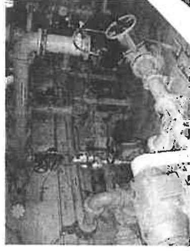
Scum Pump in Primary Gallery
