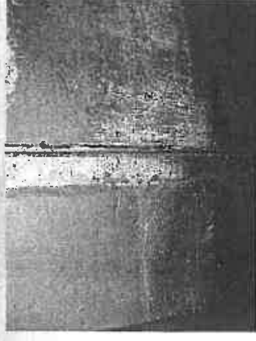
Headworks Concrete Degradation
