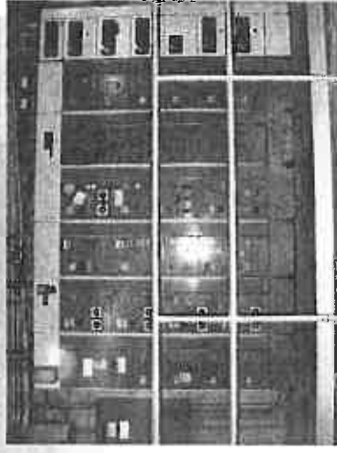
Obsolete Electrical Components in Primary Gallery
