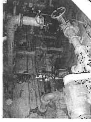
Scum Pump in Primary Gallery
