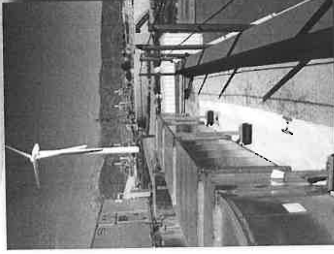
RP-4 Power Center Five Duct and A/C Access
