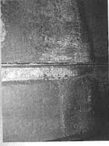
Headworks Concrete Degradation
