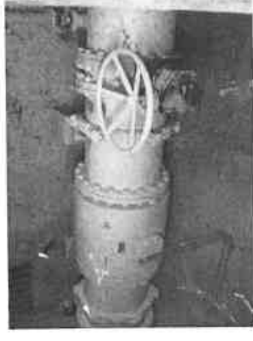
System C Flow Meter
