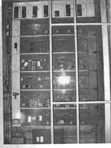
Obsolete Electrical Components in Primary Gallery
