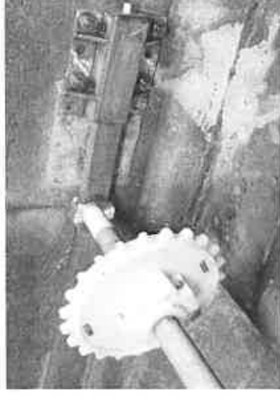
Clarifier Chain Tension Arm and Sprocket
