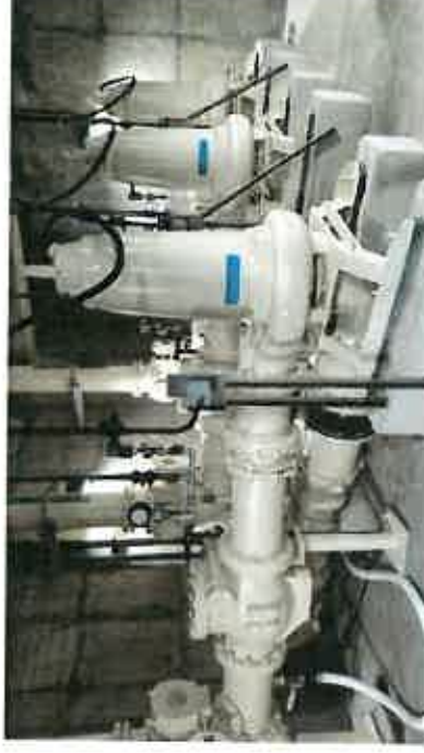
Montclair Lift Station Pumps
