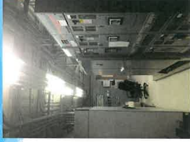
RP-5 Power Center No. 3
