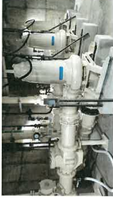
Montclair Lift Station Pumps
