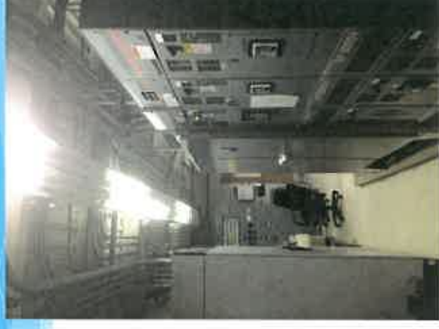
RP-5 Power Center No. 3
