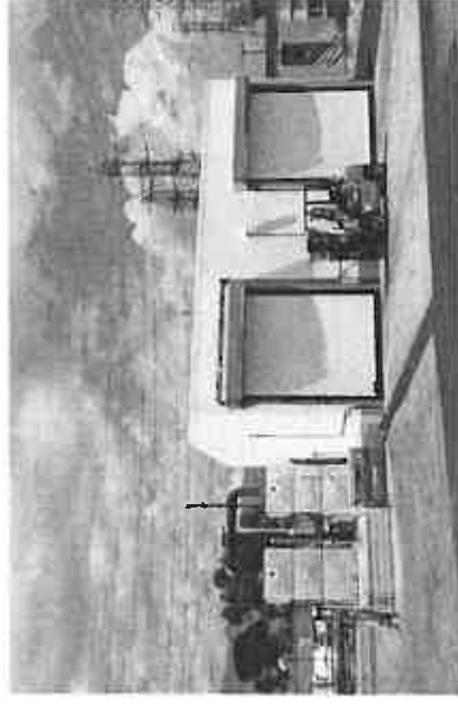
New Headworks Building and Fine Screens
