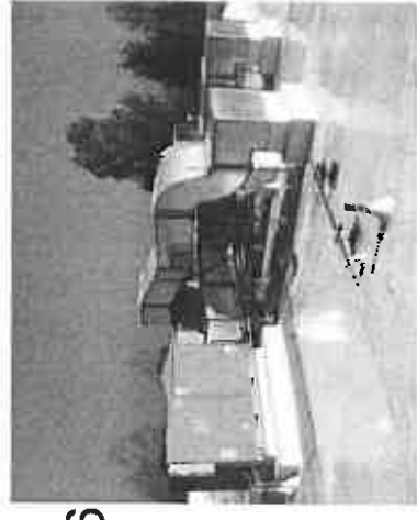
RP-5 Control & Server Rooms HVAC
