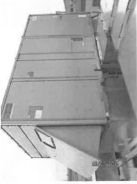
New AC unit at RP-4 MCC Bldg.
