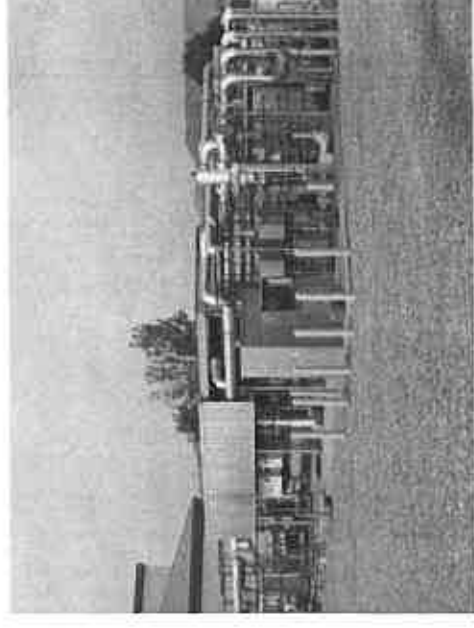
Central Chiller Plant
