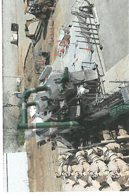
Completed Headworks Equipment
