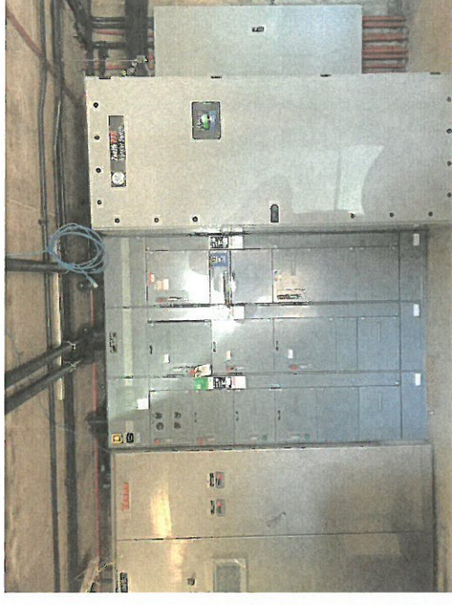
Montclair New Electrical Panel
