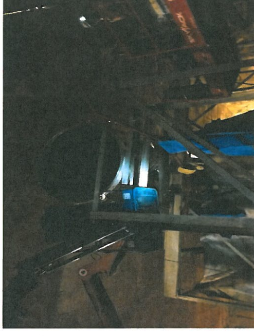
Main Dust Collecting Header
