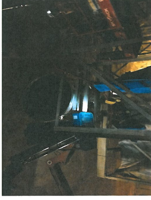
Main Dust Collecting Header
