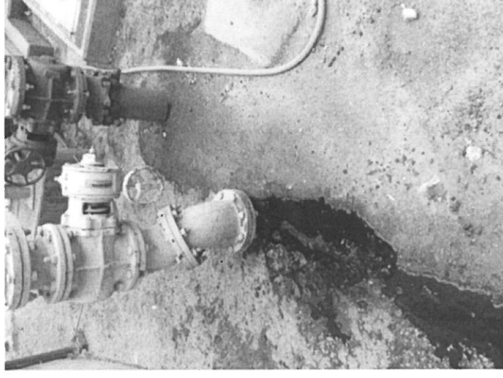
6-inch Sludge Line Leak
