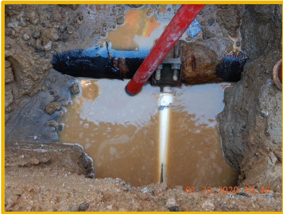
Located Broken Pipe
