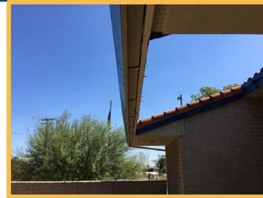
RP-1 Ops Building: Rotted Fascia
