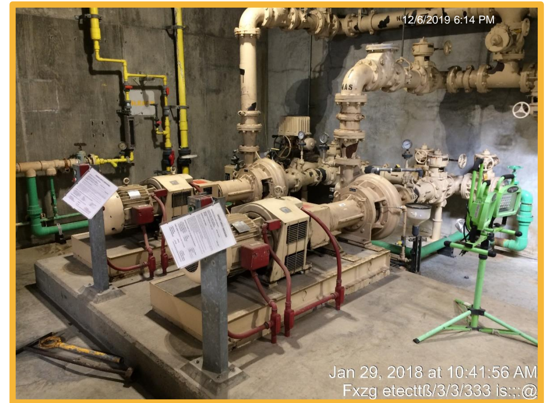
Waste Activated Sludge Pumps
